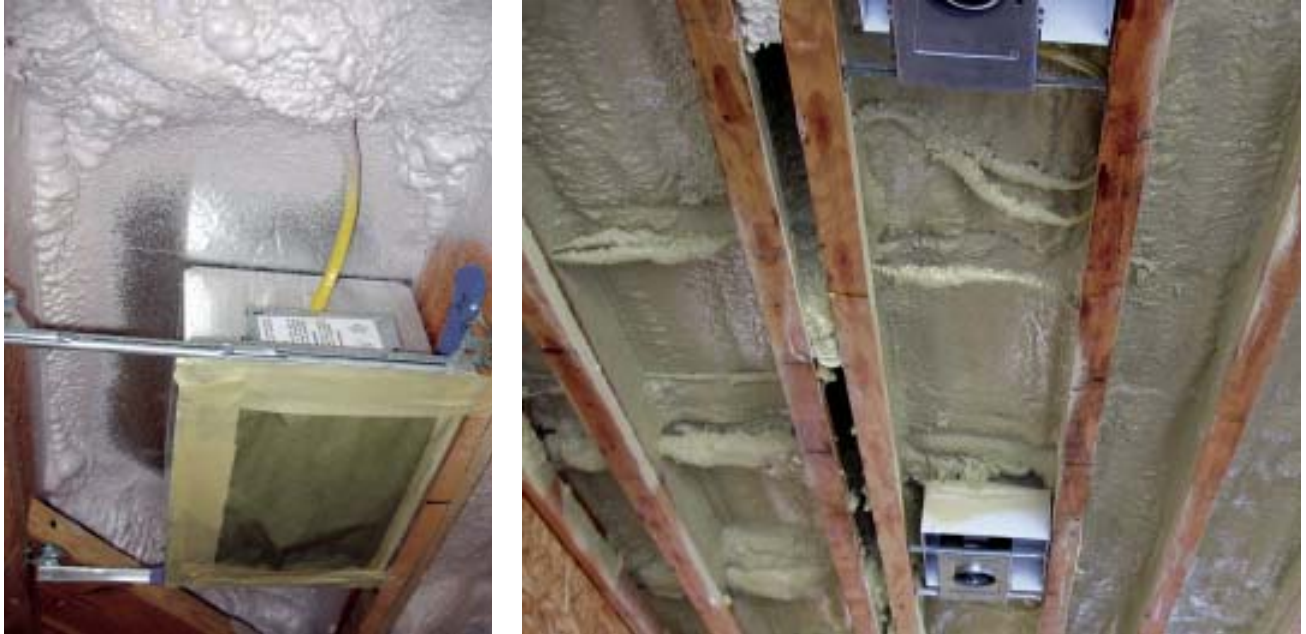
Figure 7. Code requires that a space be left between can lights — even IC-rated cans — and spray foam insulation. In shallow bays, the author’s crew installs foil-faced rigid foam above fixtures and creates a seal by lapping the spray foam onto it (left). An alternate method, which may soon be required in California, is to isolate fixtures from the foam by installing them in metal boxes (right).
