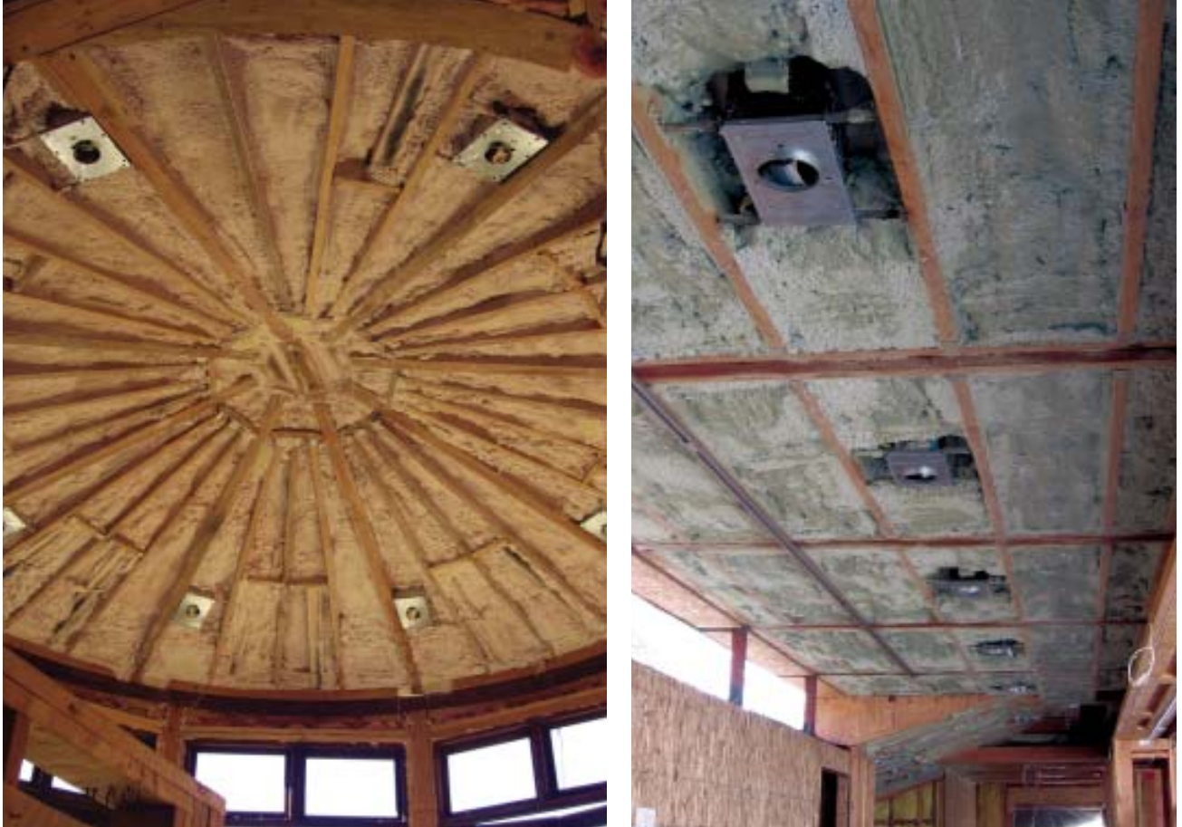
Figure 1. Spray foam is a good choice for roofs that are difficult to vent, like a turret with converging rafters (left) or a flat roof with its rafters hung between flush beams (right).
