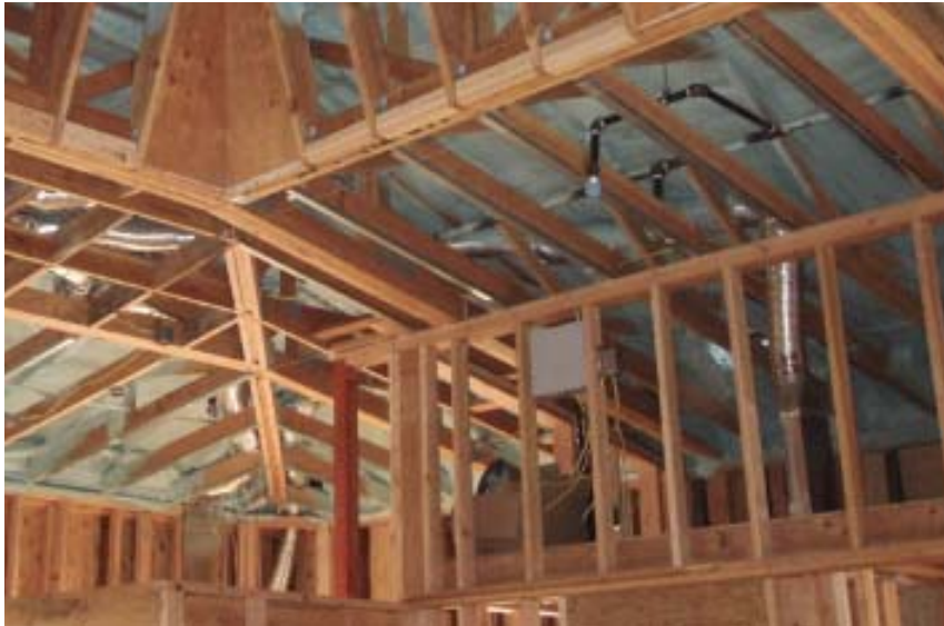
Figure 3. The ducts visible in this unvented attic will be concealed after drywall is installed. But because they are in conditioned space, they won't be subject to the extremes of temperature typical of attics.
